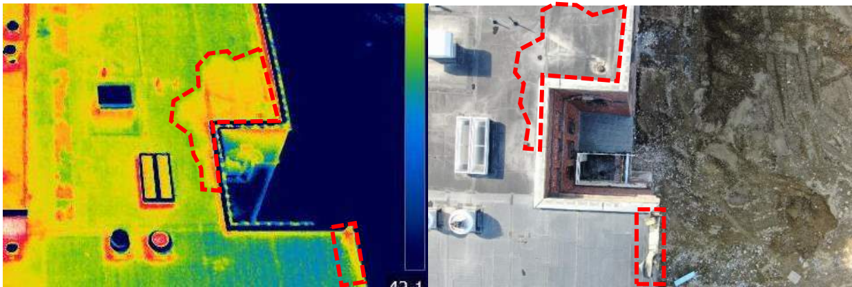
Figure 14. IR image (left) and visual light reference image (right) of thermal anomalies near drain and northeast roof edge where the roofing membrane is loose and peeled back (dashed red areas).
