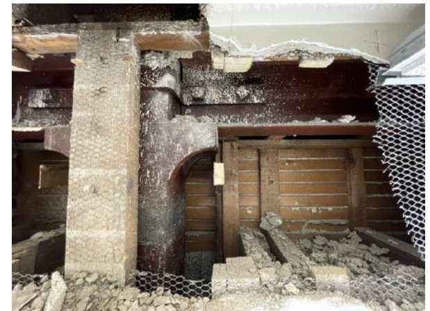
Salvaged and In-situ (from top to bottom): 1929 A-Wing facade with decorative elements; 1895 Building rosette, cast iron column
