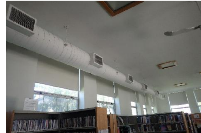
Exposed ductwork fed from rooftop air handling unit
