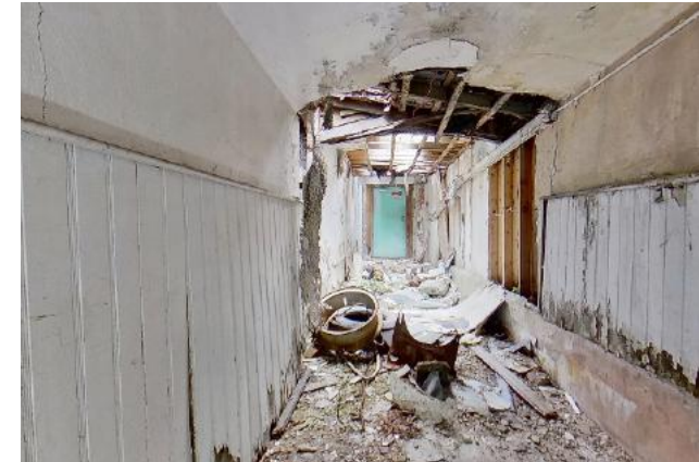
Collapsing "Office" wing constructed in south alley
