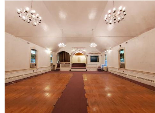
Sanctuary, with uneven flooring, cracked plaster ceiling
