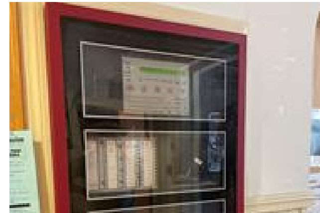
Notifier Fire Alarm Panel
