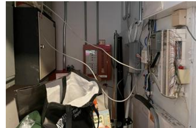
Miniscan Fire Alarm System
