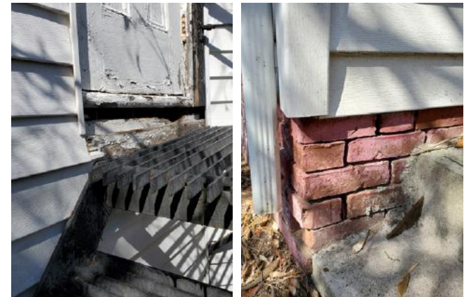
Rear entry door sill deterioration, condition of masonry foundation
