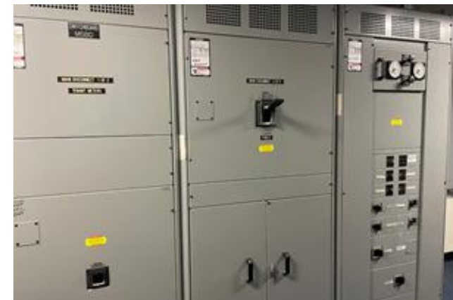
Main electrical service switchgear
