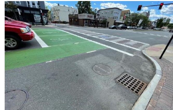
Catch basin and sidewalk on Broadway fronting building
