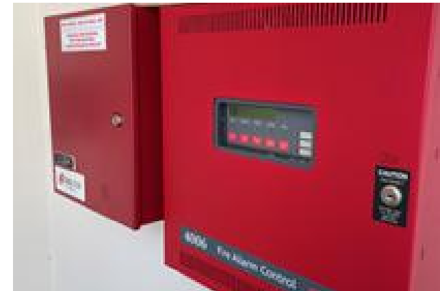
Simplex Fire Alarm System
