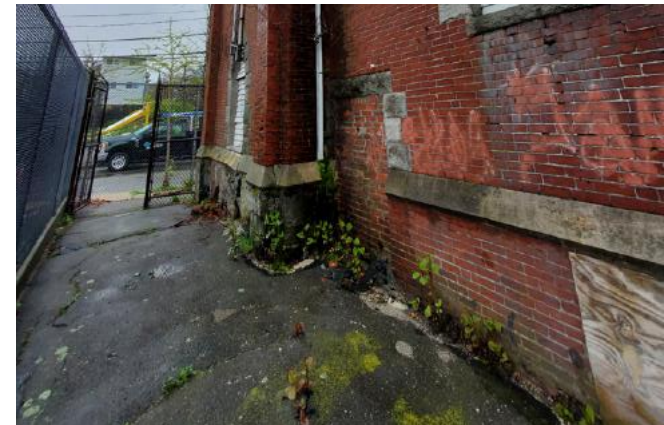
Severe weathering and displacement, brick and stone masonry at buttress
