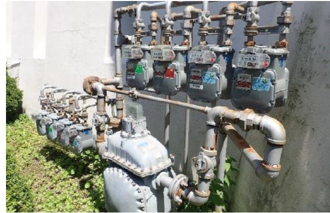
Gas meters on west side of building
