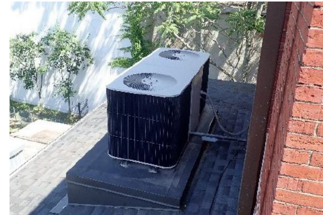
HVAC: Condensers for split DX air handling units
