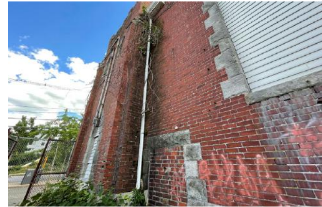
Detached aluminum downspout and bio-growth, north facade
