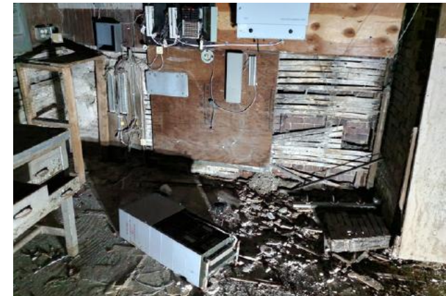
First Floor, northeast corner; electrical and telephone services and panels
