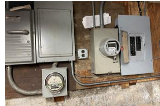
Electric service, meters and panel
