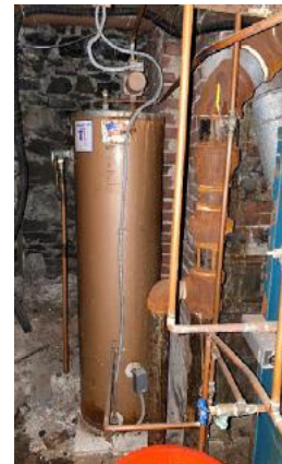
Electric hot water tank
