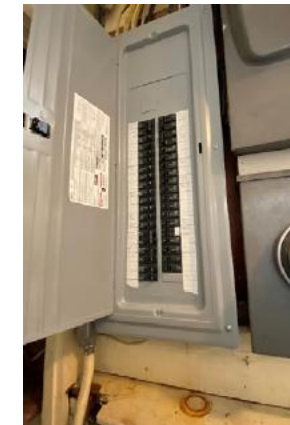
Main electrical distribution panel
