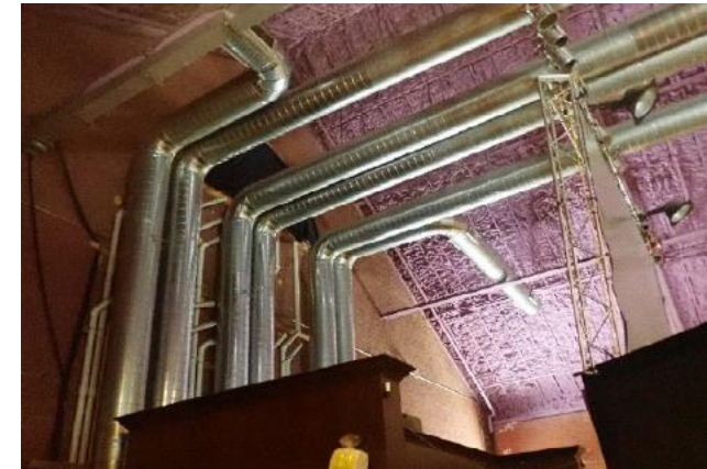
Ductwork (dating to 2009) in the Drill Hall
