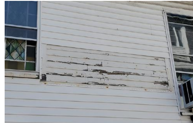
Area of prior vinyl siding loss or removal; wood clapboards exposed
