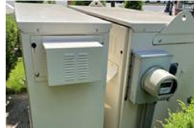
Pad-mounted transformer, west elevation
