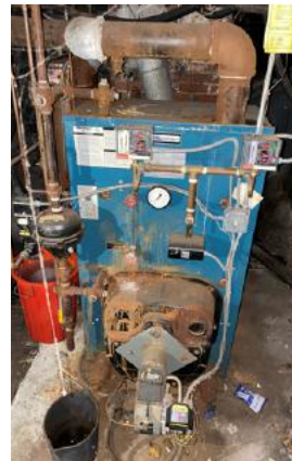
Oil-fired boiler and oil tanks, Sub-Basement
