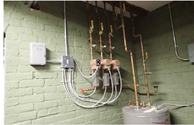
Domestic hot water heater and recirculating pumps
