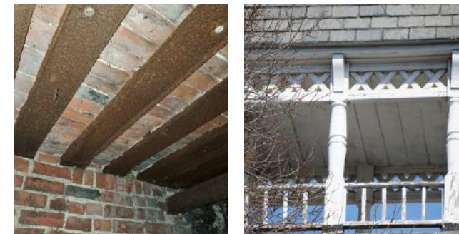
Evidence of moisture in the Sub-basement, open steeple belfry
