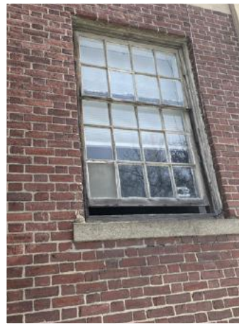
Window in poor condition
