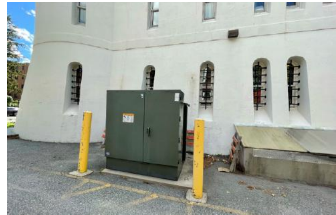
Pad-mounted transformer and plastic areaway cover at southeast corner
