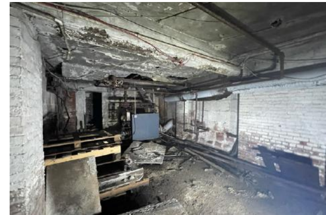
Basement with defunct boiler
