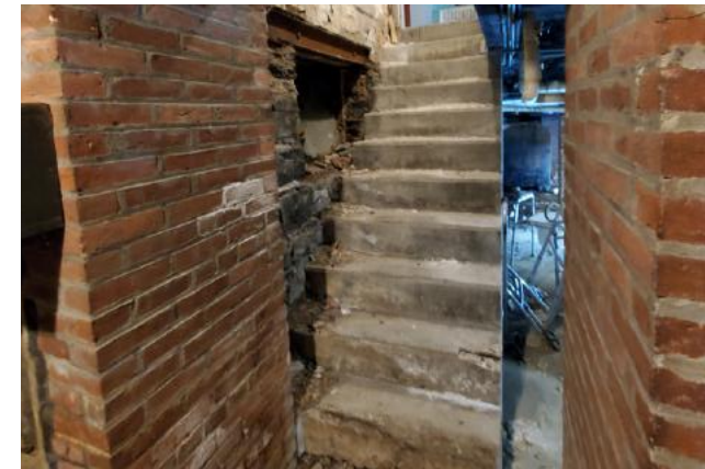
Basement; concrete basement Stair in poor condition
