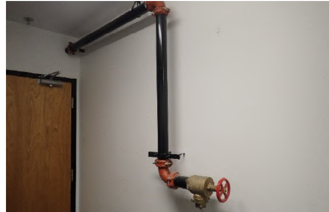
Sprinkler control valve assembly
