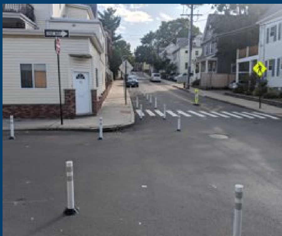
Flex posts installed to provide quick-build bumpouts and pedestrian safety benefits while construction projects are planned
