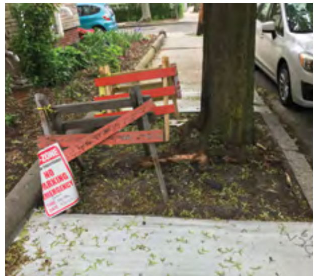
This photograph is a good example of root damage that can occur when a sidewalk is replaced. Some roots were cut and others were stripped when the old sidewalk was removed. This is an issue because these critical, anchoring roots have now been damaged and may not recover.
