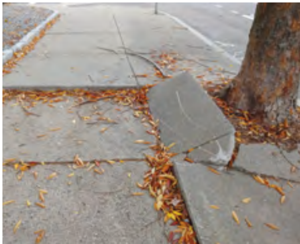
This Japanese zelkova along Broadway is causing significant uplift of the sidewalk.
