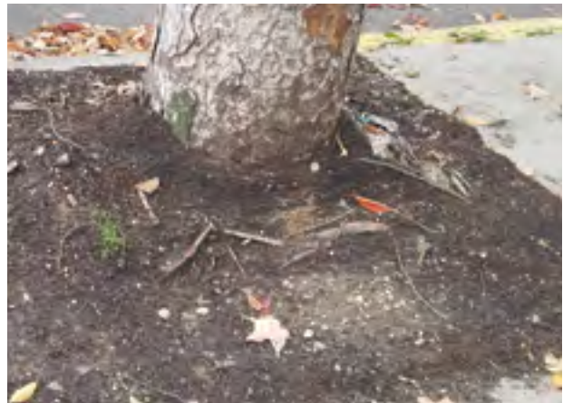
The tree above has no visible root flare, indicating it was planted too deep.
