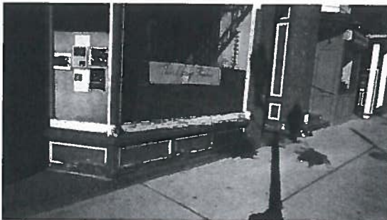
Deteriorated Plywood Base Sheathing
