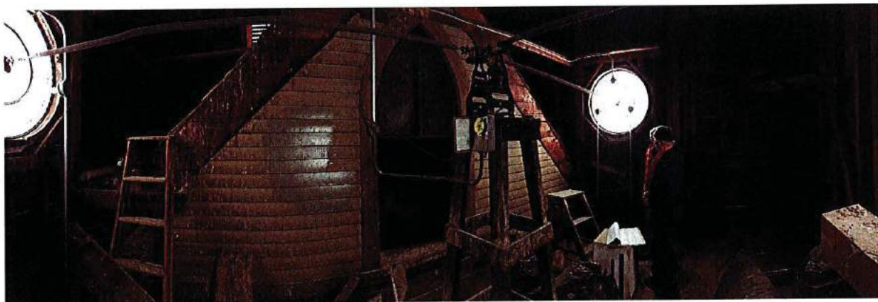
7 Panorama view of the interior of the clock tower showing the end gable of the original church. The geared mechanism to run the clocks is to the right of the ogee window. Note also the crossed-braced framing in the exterior walls.
