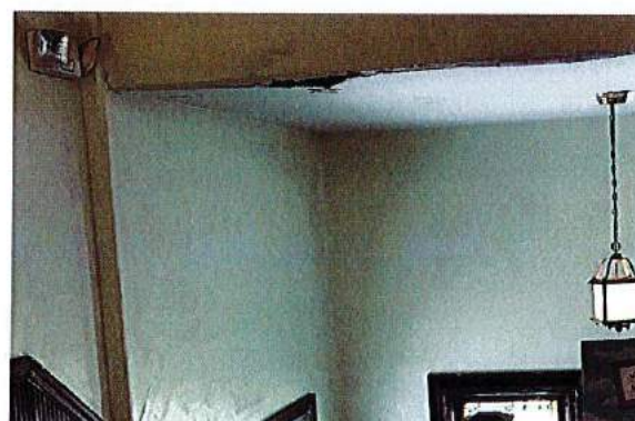
3 Roof-wall intersection and possible leak above the north stair.
