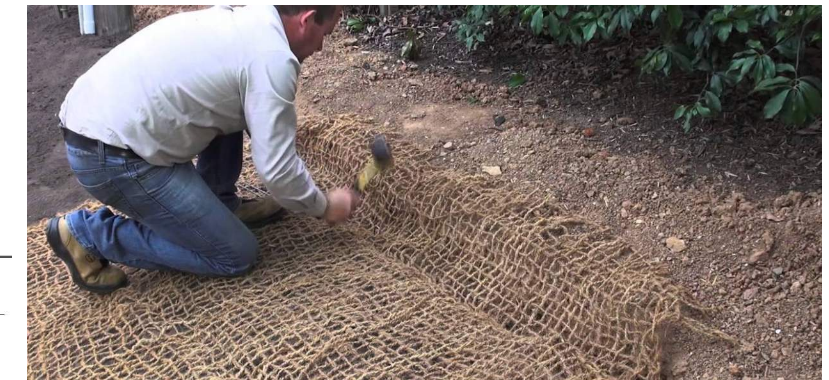
Above: Install Coir Mat to Stabilize Slope and protect new plants and seeds from washing away
