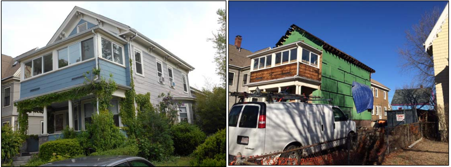
139 Summer Street – Left photo is prior to building permit while the right photo is after
