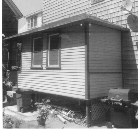
After photo showing enclosed porch (area below porch has since been screened with lattice)
